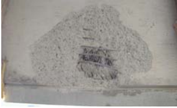
Figure 2: Failed anchorage in slab edge photographed on construction site
