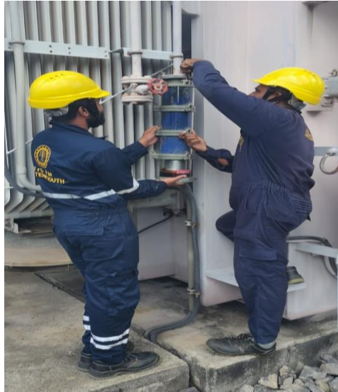
Figure 4.4 Breather at Madampe Transformer 02
