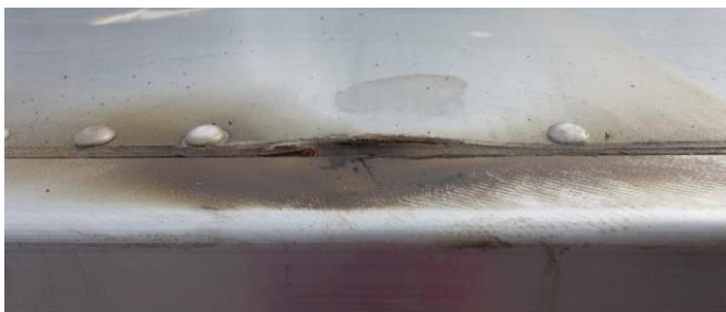
Figure 5-10: AKE container roof damages
