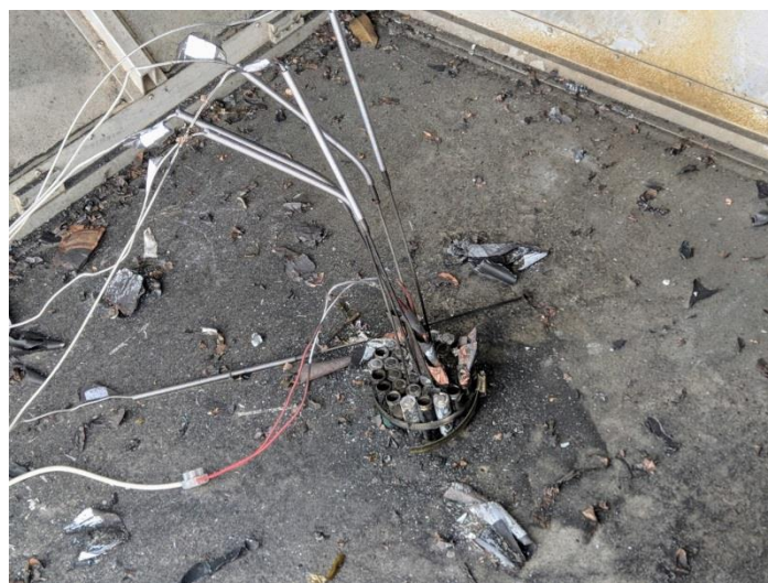
Figure 5-1: Battery thermal runaway post-test
