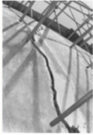
Cracks on the dome
