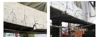
Debonding & Cover delamination
