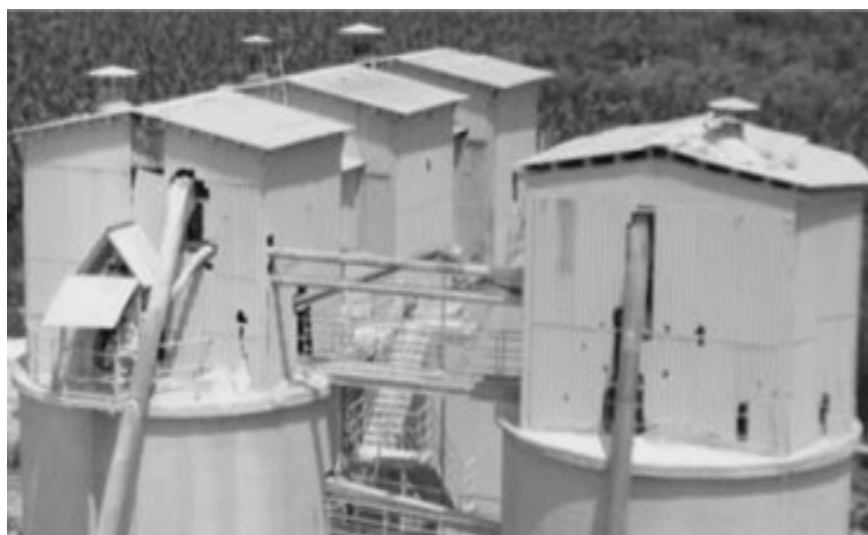
Figure 2-17: Mini dust bag system on blending silos at HLL – PCW
