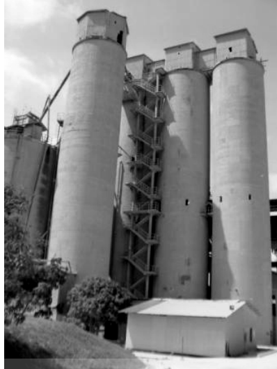
Figure 2-9: Homogenizing silos (blending silos) at PCW
