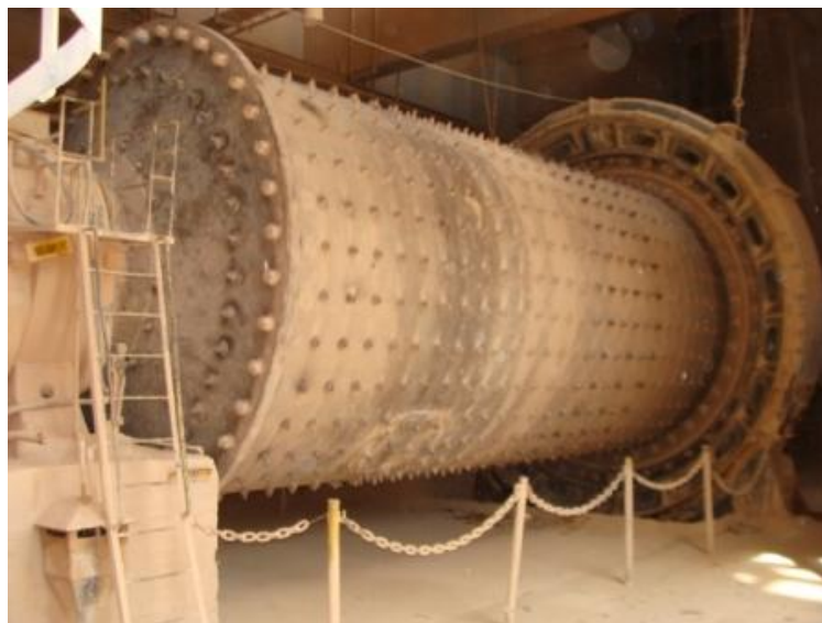
Figure 2-8: Raw mill at HLL – PCW
