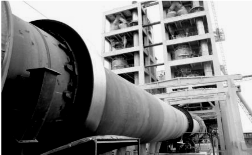
Figure 2-12: Clinker kilns & pre-heater tower at HLL - PCW
