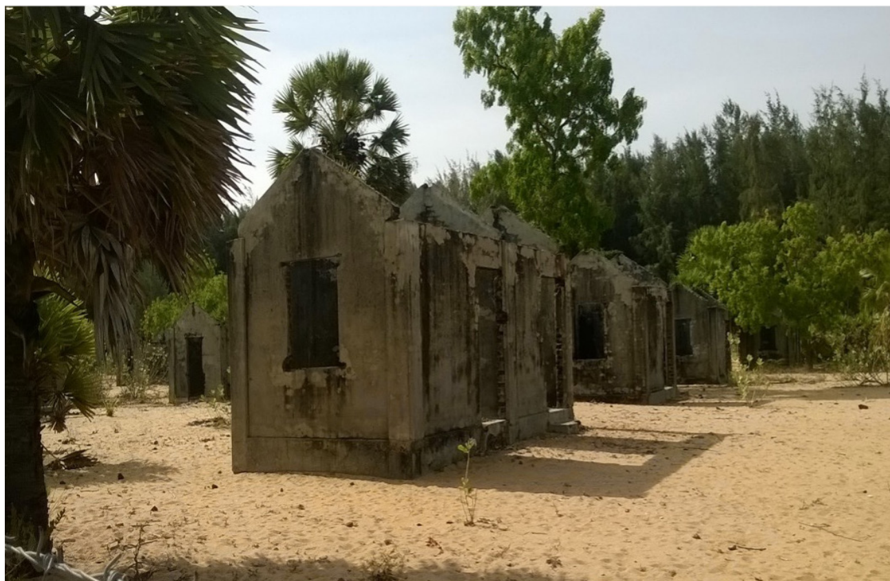
Figure 2 : An abandoned incomplete resettlement housing scheme, Batticaloa, Sri Lanka
