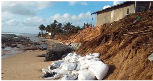
Figure 9 - Coastal erosion due to Natural impacts
