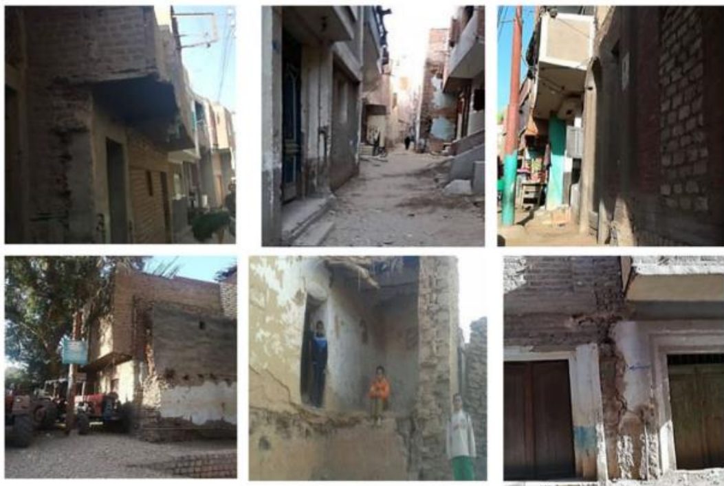
Figure 11 : Improper maintenance of CSEB buildings
