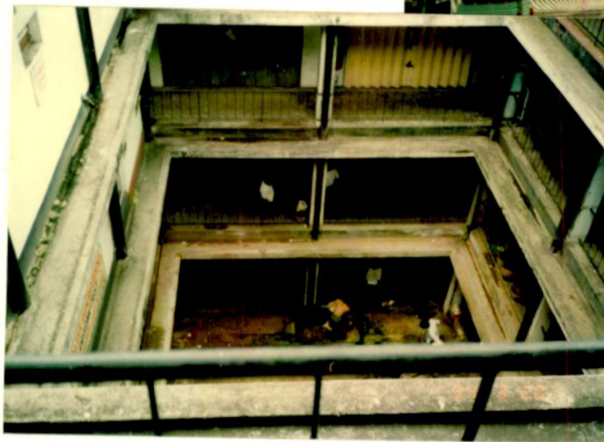
(Fig. 32 b ) Borella supermarket Underused, a design failure.
