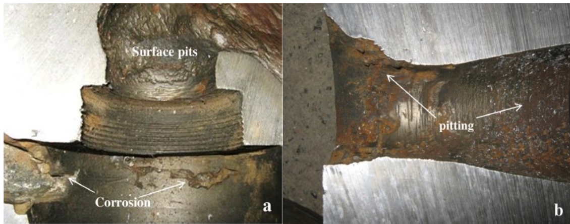
Figure 2.6: corroded inner surface of the control valve body, (a) near the seat ring and (b) near the valve's flange [28]
