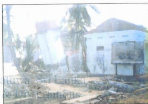
Fig 2.7 A completely damaged House at of Saudhapuram.
