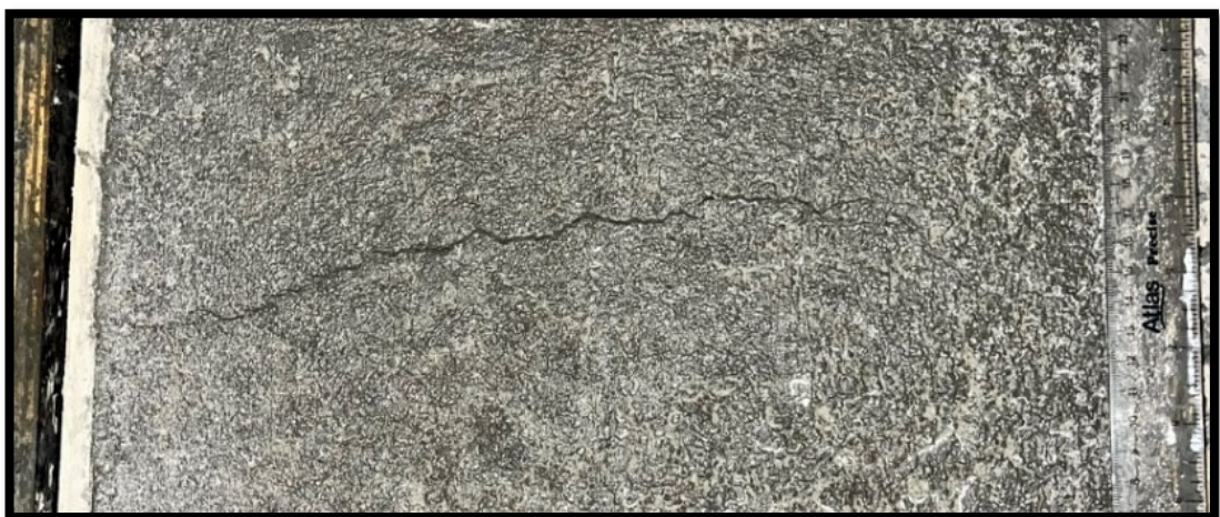
Figure 4.13 : 150% enlarged view of the crack
