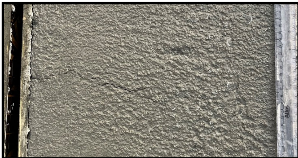
Figure 4.9: 150% enlarged view of the crack
