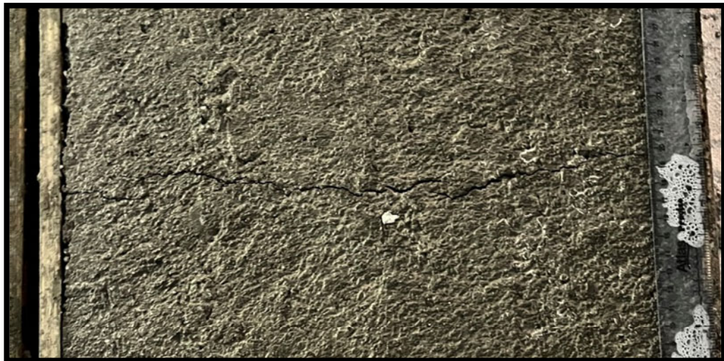
Figure 4.7: 150% enlarged view of the crack
