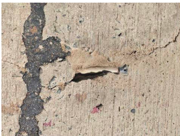
Figure 2: Joint Spalling and Cracking
