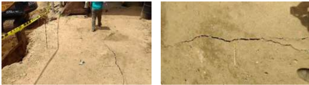
Figure 2.6: Initiation of Ground Cracks.
