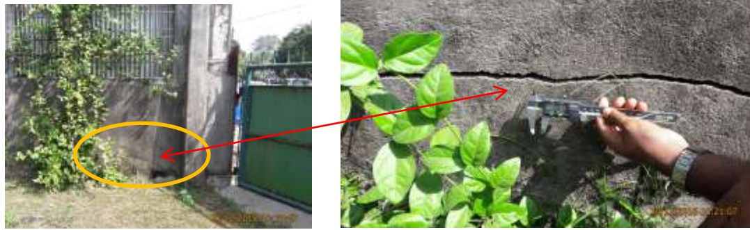
Figure 2.19: Separation of boundary wall of T13 House.
