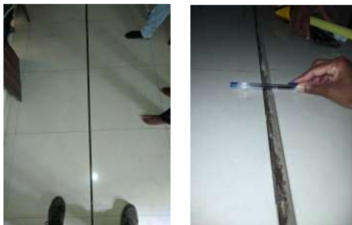
Figure 2.11: C5 floor crack.
