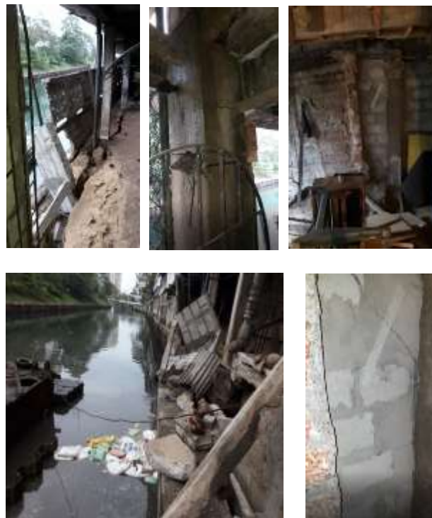
Figure 2.32: Photographs of cracks in the lower basement.
