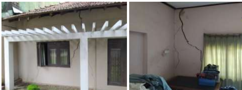
(a) C1 crack outside view
