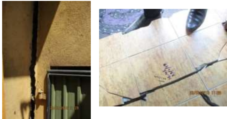
Figure 1.1: The nature of wall and floor crack of a building.
