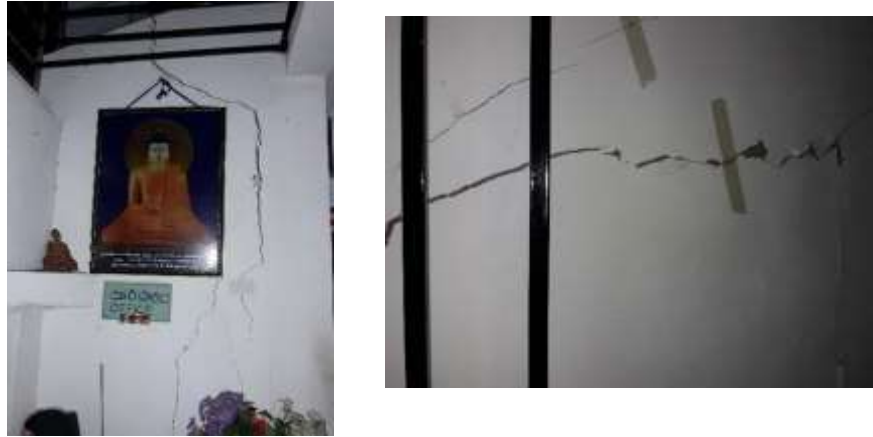
Figure 2.33: Photographs of cracks in the upper basement.
