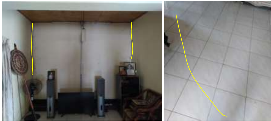
(a) C2 wall crack
