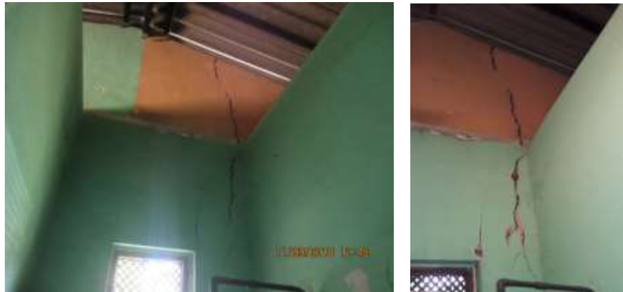
Figure 2.24: C4 crack on 11.09.2018 and 19.12.2018.
