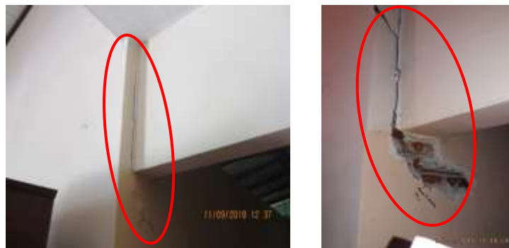
Figure 2.22: C2 crack on 11.09.2018 and 19.12.2018.
