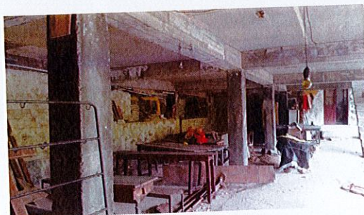
Figure 9 - Slight spalling of concrete in columns
