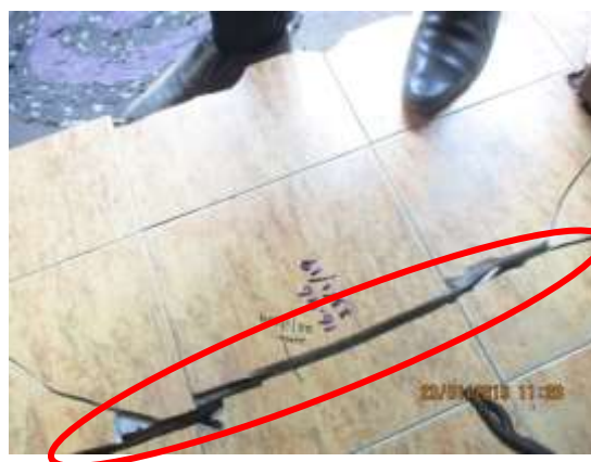
Figure 3.12: C1 floor crack.
