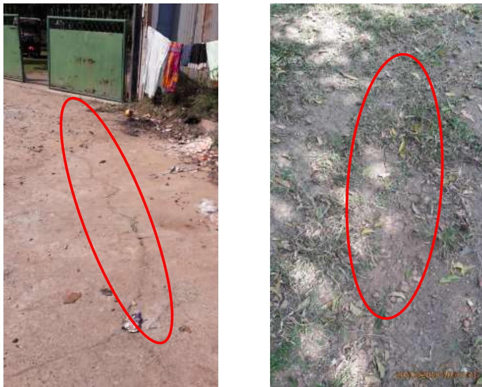
Figure 2.18: Ground Cracks at front side of T13 House.
