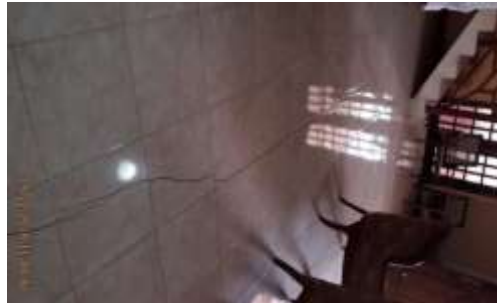
Figure 2.21: C1 crack on 19.12.2018.
