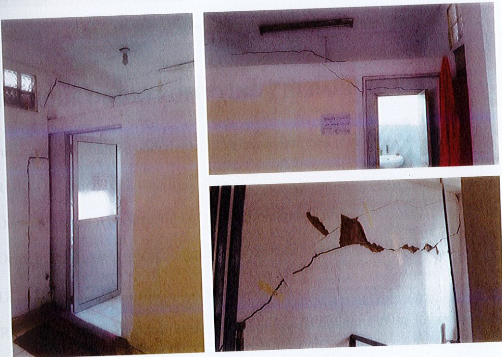
Figure 11 - Cracks observed in upper basement wash room walls
