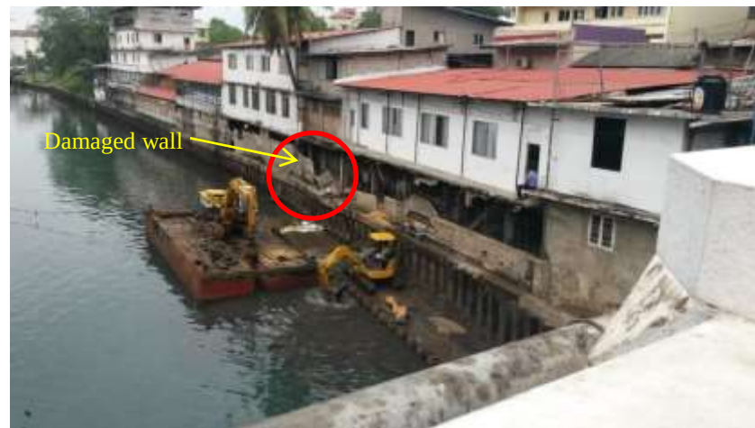
Figure 2.31: Location of canal bank instability initiated.
