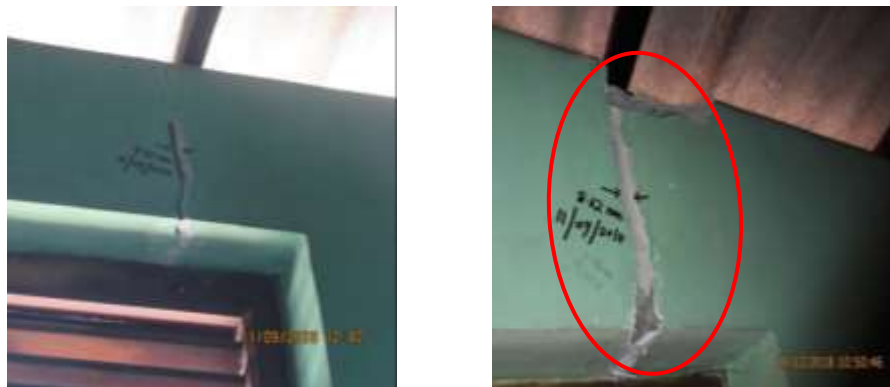
Figure 2.23: C3 crack on 11.09.2018 and 19.12.2018.
