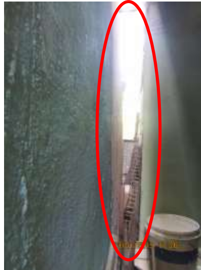
Figure 3.9: Detachment – 2 observed in the wall.
