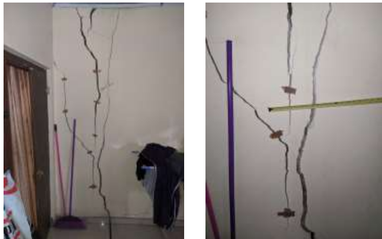
Figure 2.9: C2 and C4 cracks.
