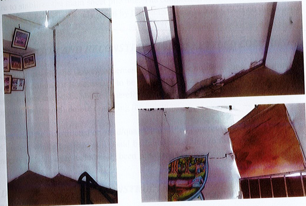
Figure 12 - Shifted walls and slabs observed in the ground floor
