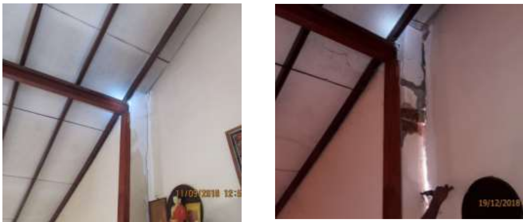
Figure 2.25: C5 crack on 11.09.2018 and 19.12.2018.
