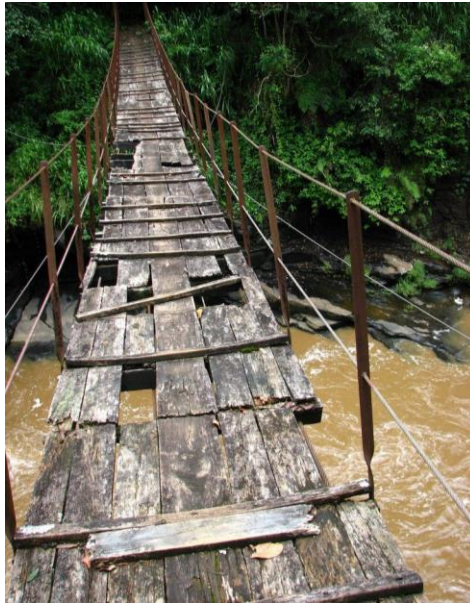
Figure 3.2: Old pedestrian bridge in poor condition in Kothmale
