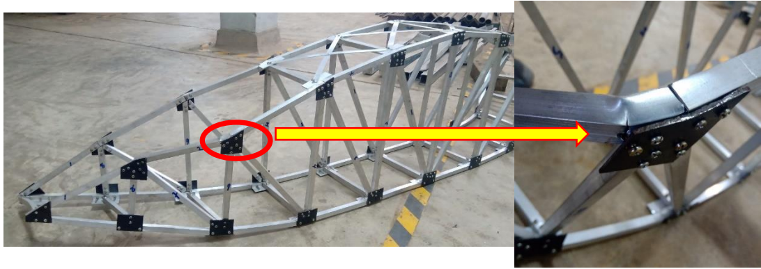
Figure 5.21: Initiating point of the crack of truss A
