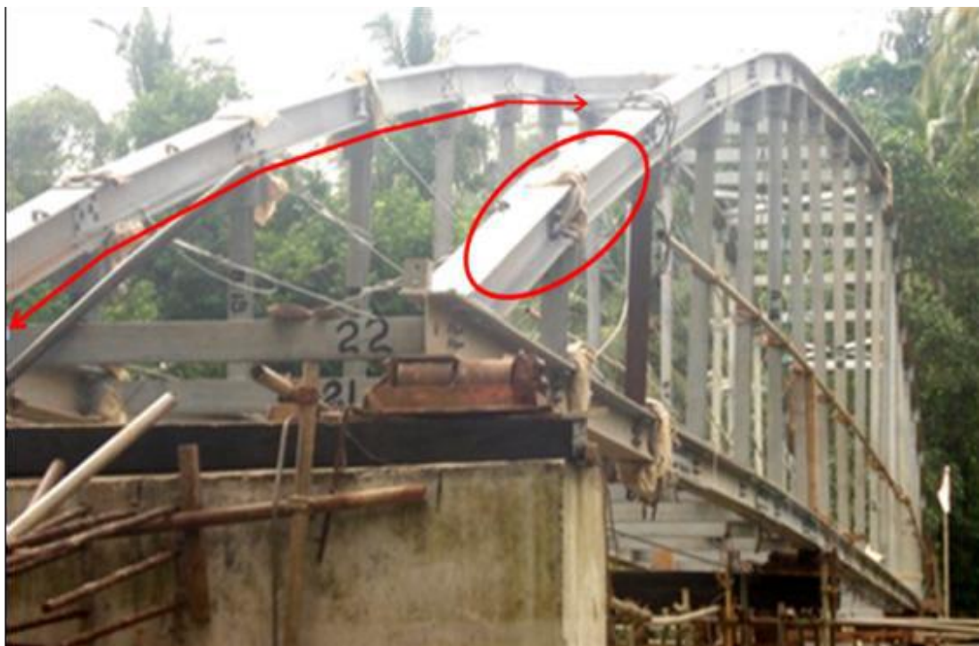
Figure 3.16: Failed Ehalakanda Bridge when launching
