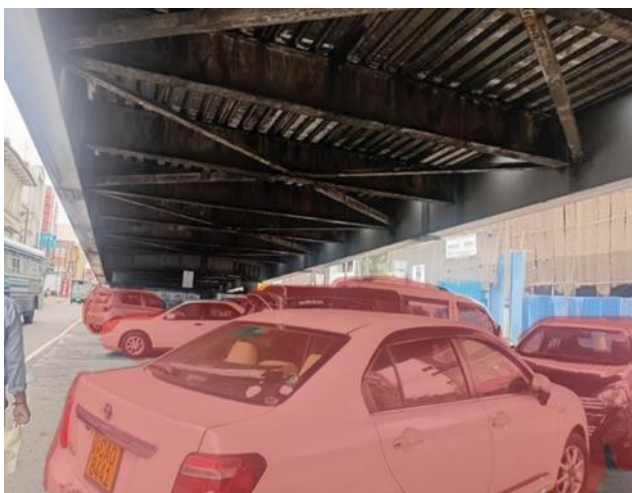
Figure 6 Irregular Vehicle Parking (Author)
