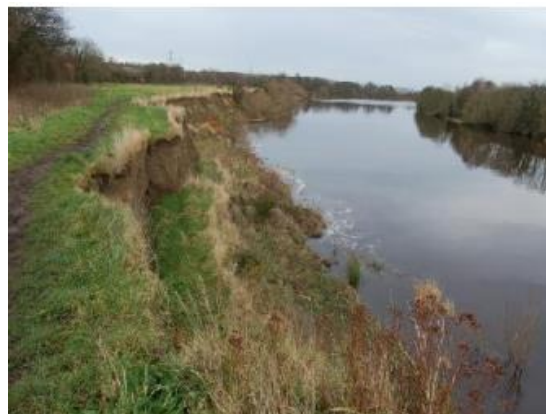
Figure 2.4 Photograph illustrating how turbulent water currents can cause embankments to break.
