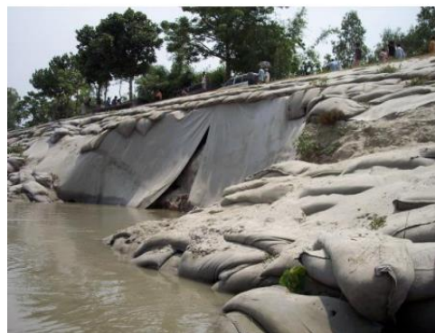
Figure 2.14 Cyclonic Storm Surge Protection: The Poor Performance of Sand Bags
