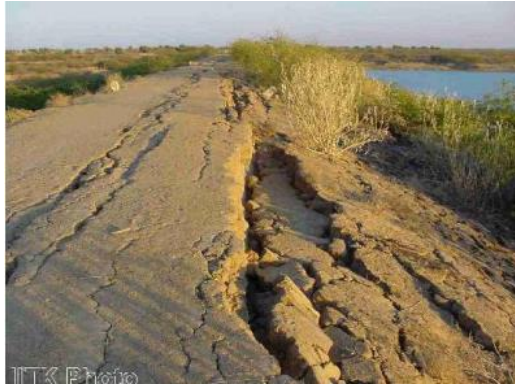
Figure 2.1 Failure of road Embankment
