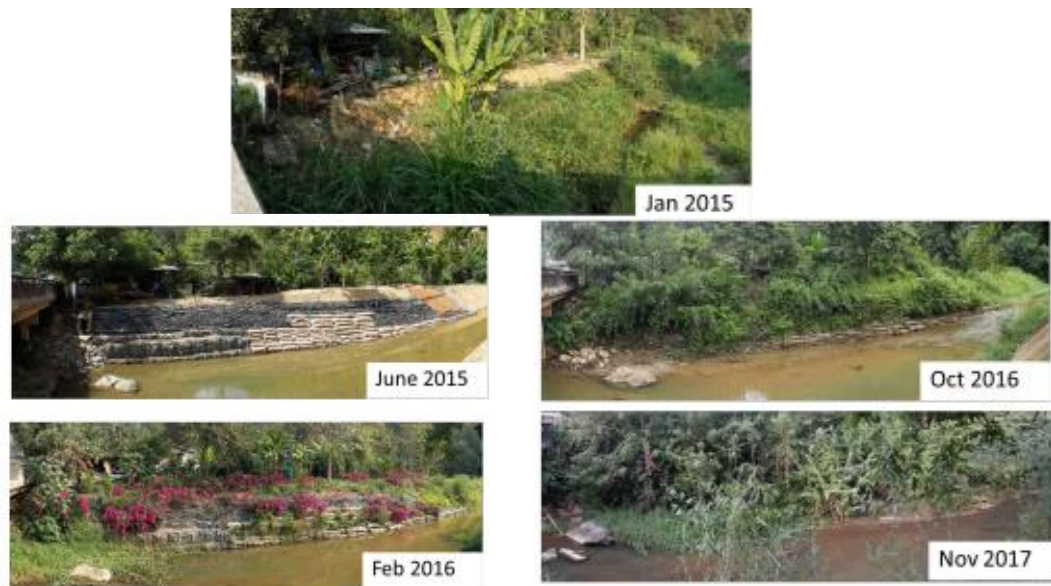
Figure 2.13 Appearance of the vegetation cover of the failed sections over time
