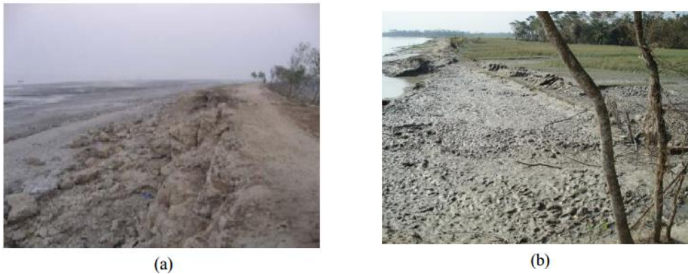
Figure 2.3 Photographs ‘a’ and ‘b’ depict embankment damage brought on by wave action
