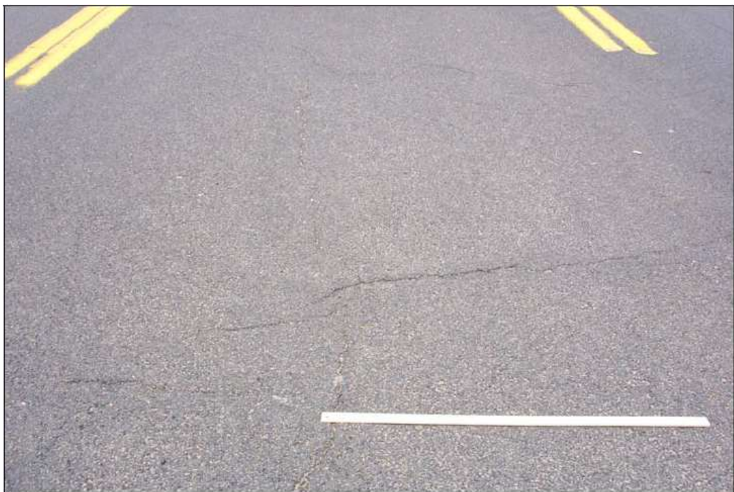
Figure 3.21: Low Severity Alligator Cracking with Few or No Interconnecting Cracks (Federal Highway Administration, 2006)
