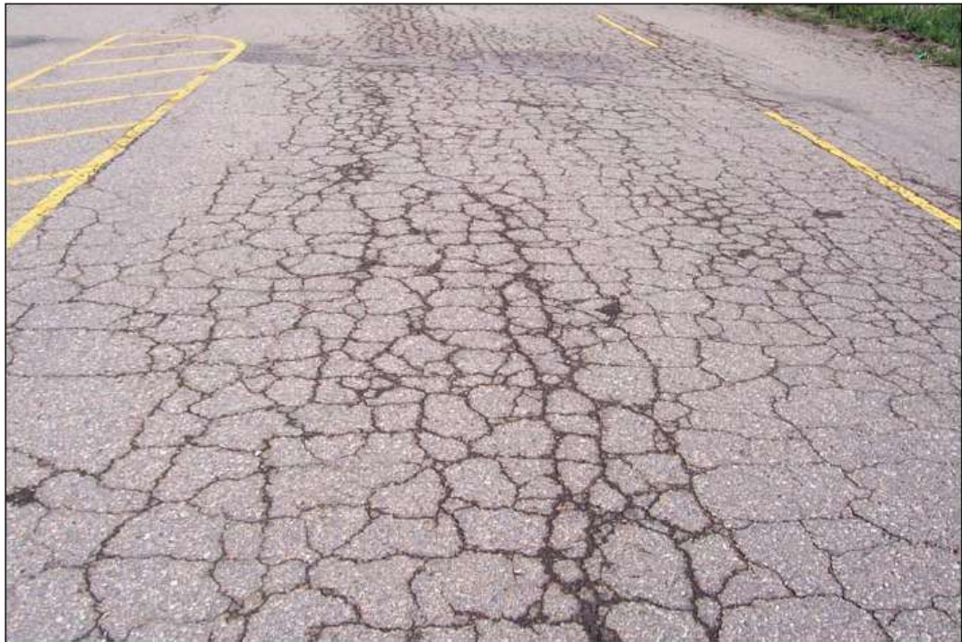
Figure 3.19: High Severity Alligator Cracking (Federal Highway Administration, 2006)
