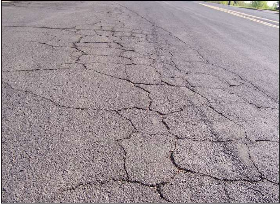
Figure 3.20: Medium Severity Alligator Cracking (Federal Highway Administration, 2006)
