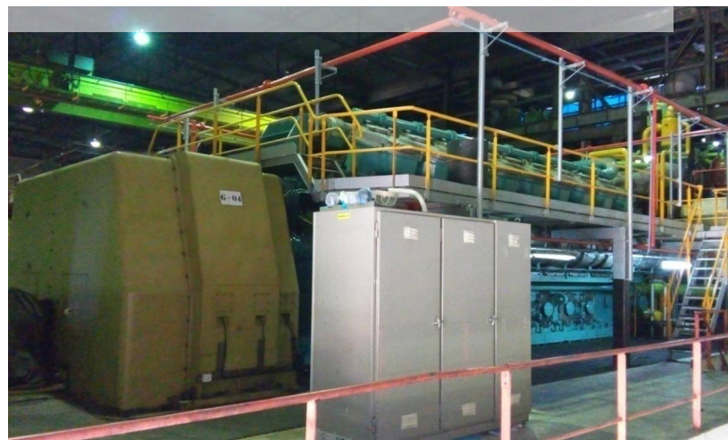
Figure 5:6 Pielstick plant generator with Diesel engine
