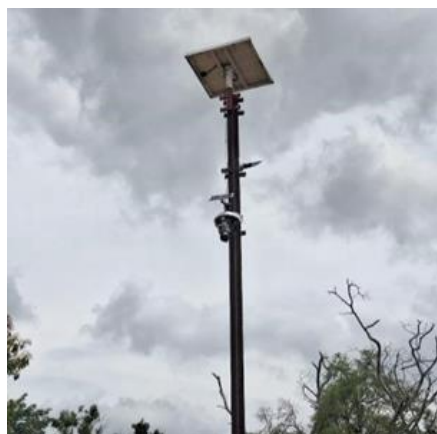
Figure 9: CCTV lighting system in Galgamuwa
