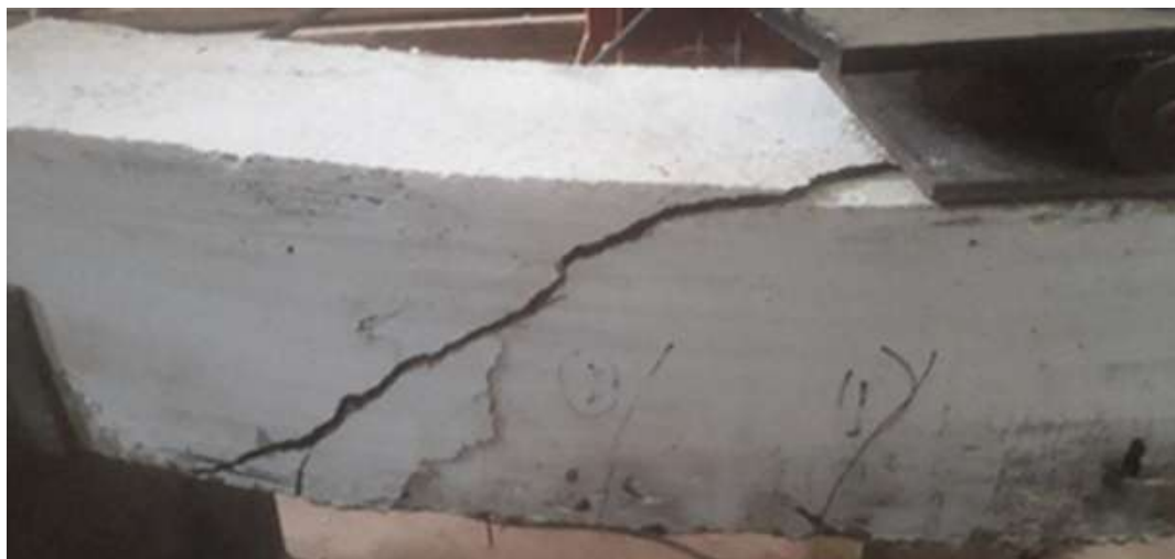
Figure 11: Cracks in a 2m radius curved beam
