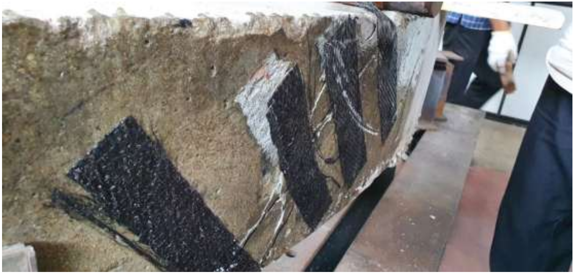
Figure 32: De-bonding of shear strips – Beam B
