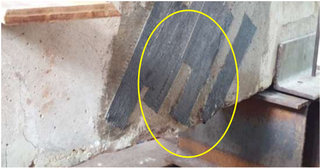
Figure 30: De-bonding of shear strips – Beam A
