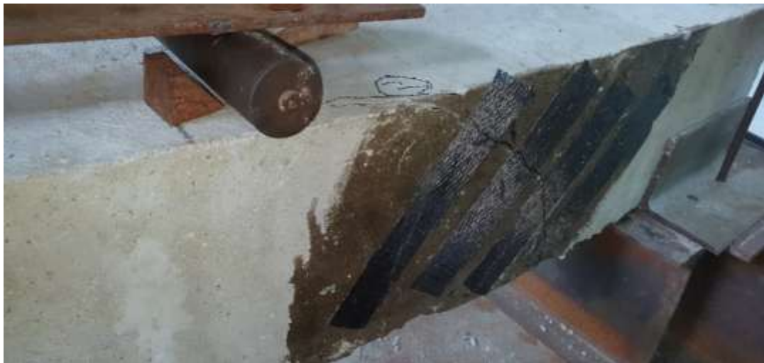
Figure 35: Shear crack propagated –Beam D
