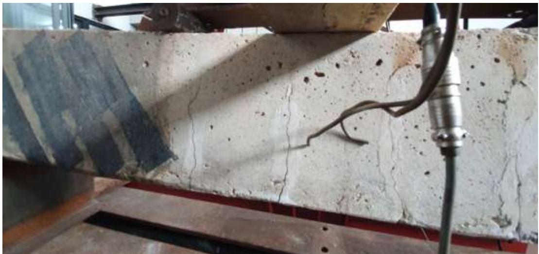
Figure 29: Flexural cracks appearing at the locations where a moderate crack repair was done – Beam A
