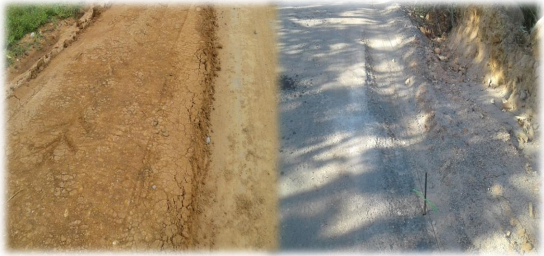
Figure 3: Some problematic area due to Sub base fail in I road Polonnaruwa
