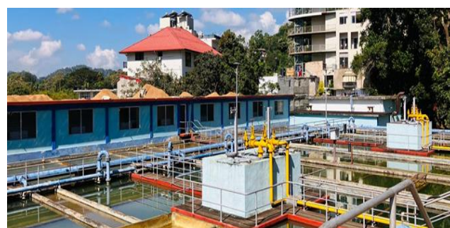
Figure 03: Pulsator Technology, Water Treatment Plant, Kandy Municipal Council.
