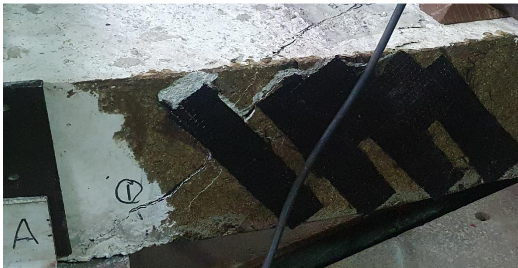
Figure 36: Shear crack induced debonding of CFRP in Beam 2-2-SS
