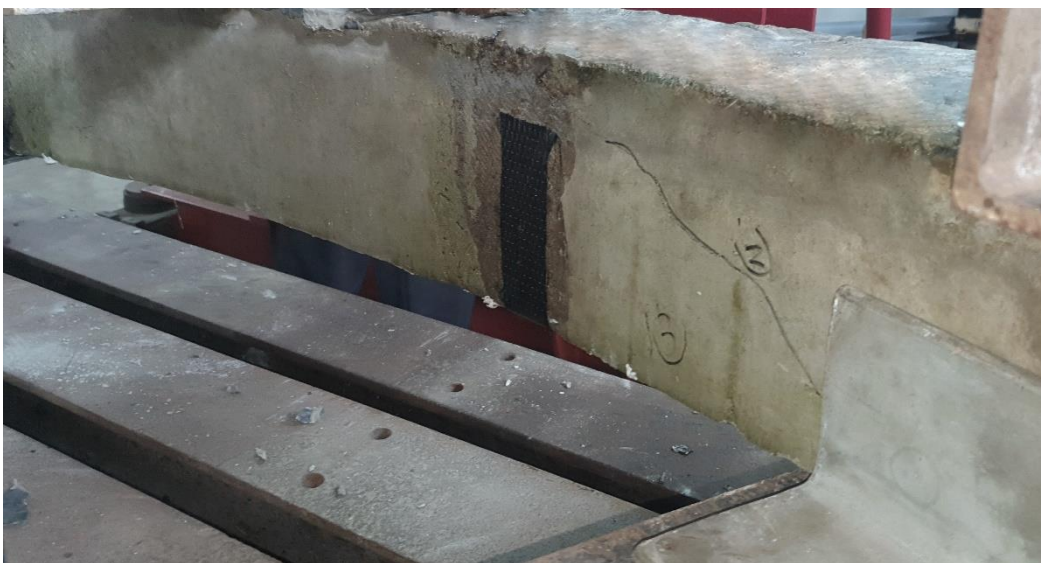
Figure 28: Cracks in a Beam 2-2-FS
