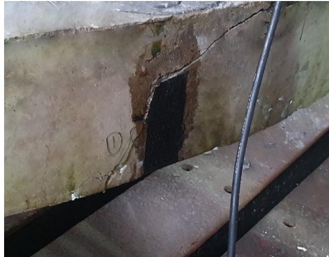
Figure 29: Shear failure of Beam 2-2-FS & debonding of CFRP fabrics
