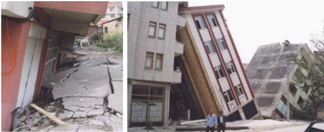
Figure 3.3: Typical examples of bearing capacity failure in the city of Adapazari during the 1999 Kocaeli earthquake. Adapted from (Yilmaz et al., 2004)
