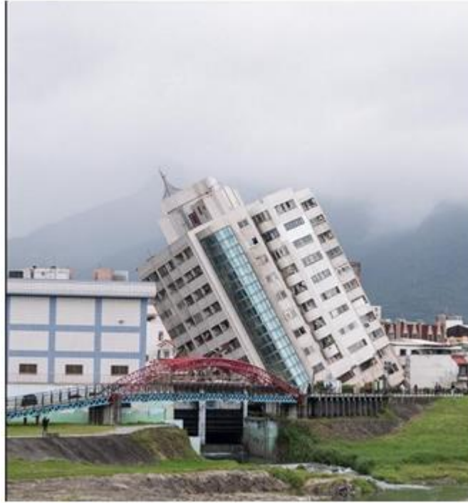
Figure 3.2: Collapsed an apartment building after reaching the ultimate limit state of the sub-soil, Taiwan 2018.
