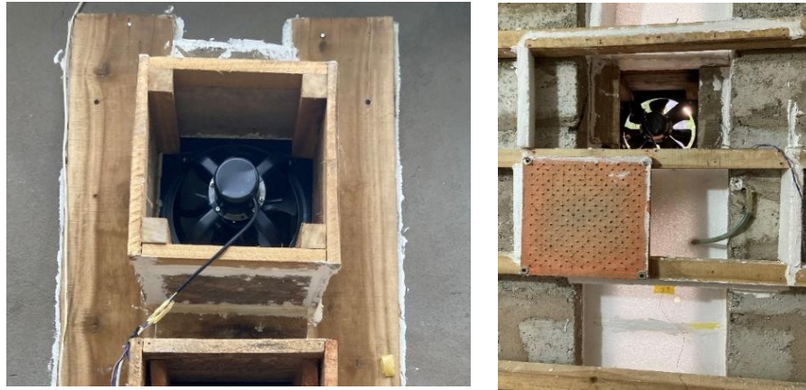
Figure 5-10: boxed DC fan is fixed to the primary wall from the outside, positive ventilation will be provided from outdoors to indoors
