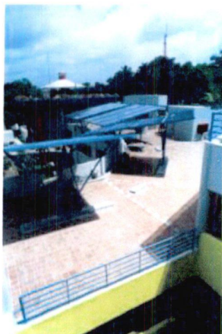
Fig 29. Solar panels placed as sun protector also –Media center, Pelawatta
