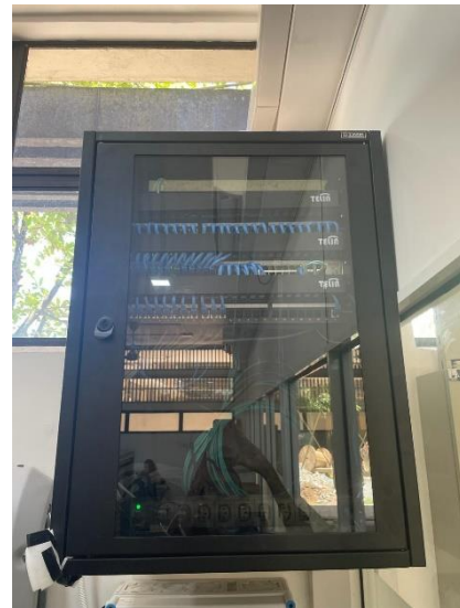
(b) Network Switch
