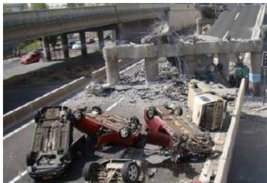
Figure 2.1. Unseating of superstructure
