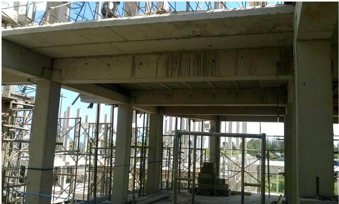
Figure 1.1 – Precast prestressed slab panels rest on beams without having falsework for slab.
