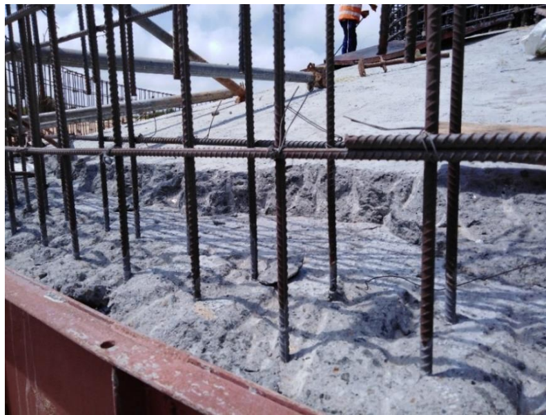
Figure 2-1 Cold Joint in top layer of the foundation (at wind power project during the construction in 2020)
