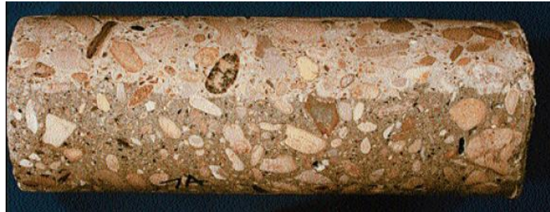
Figure 2-2 Signs of a pour lines: interface exhibits a rough surface with aggregate protruding between lifts and no voids (Volz et al., 1997)
