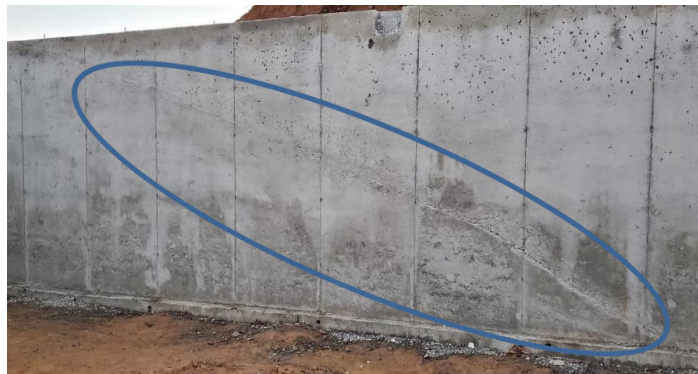
Figure 1-1 Cold Joint ( https://inspectapedia.com/ )
