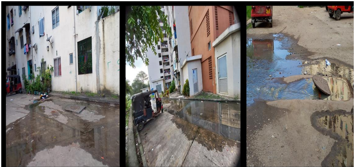
Image 4.54 – View of Sewer water flooding streets of Randiya Uyana
