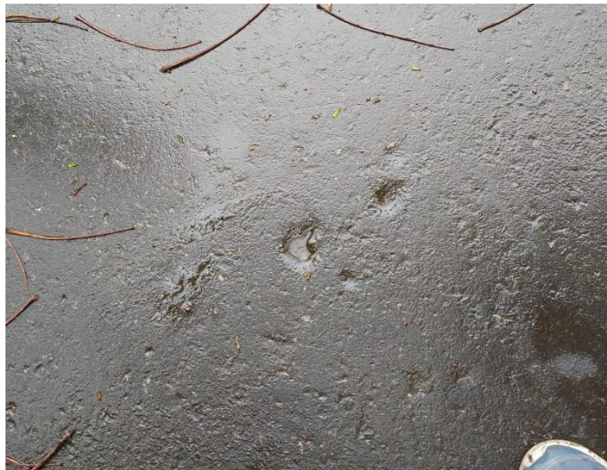
Figure 4.34: Section B - Raveling – dense mix asphalt (Low-Severity level) 7) Weathering (surface wear) – dense mix asphalt
