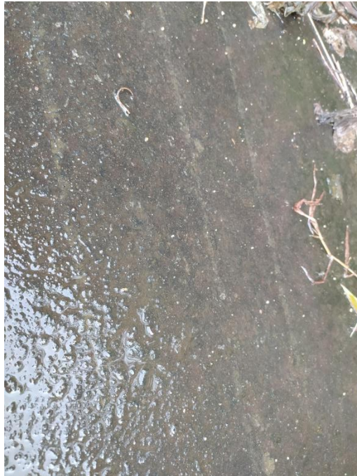
Figure 4.31: Section A- Rutting (Low-Severity level)
