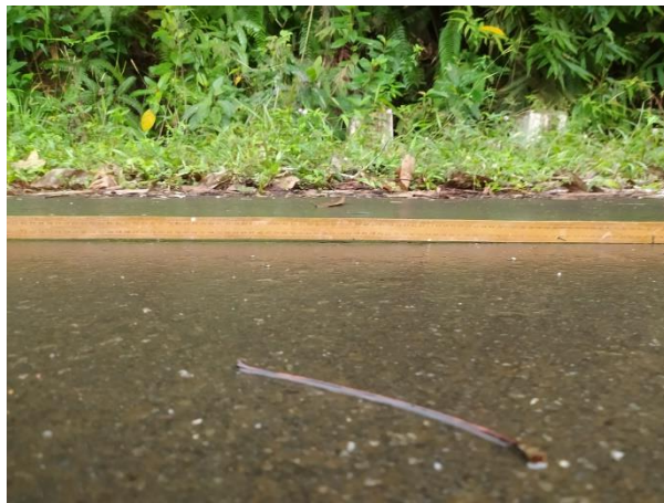
Figure 4.25: Section B – depression (Low-Severity level)
