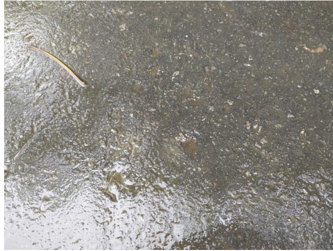
Figure 4.35: Section A - Weathering (surface wear) - dense mix asphalt (Low-Severity level)
