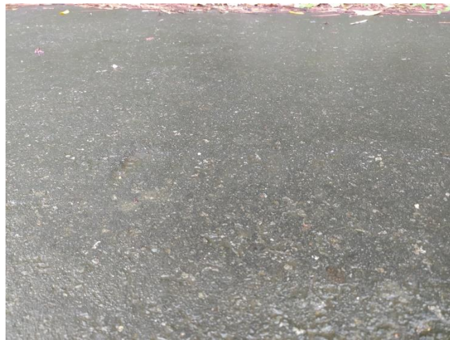
Figure 4.36: Section B - Weathering (surface wear) – dense (Low-Severity level)
