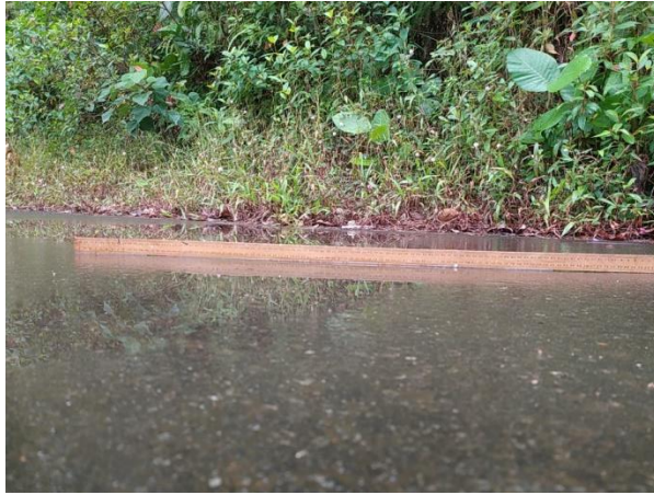
Figure 4.24: Section A - depression (Low-Severity level)
