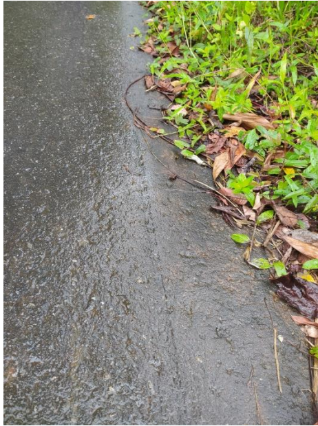
Figure 4.26: Section A- Edge cracking (Low-Severity level)
