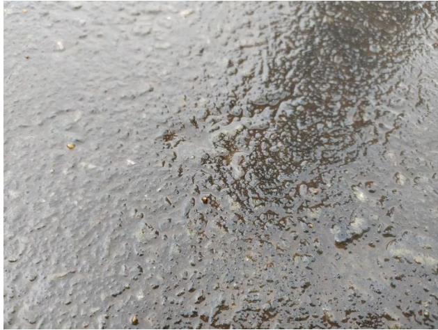
Figure 4.30: Section B- Polished aggregate (Low-Severity level) 5) Rutting
