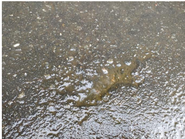
Figure 4.29: Section A - Polished aggregate (Low-Severity level)
