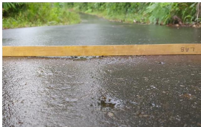
Figure 4.32: Section B- Rutting (Low-Severity level) 6) Raveling – dense mix asphalt
