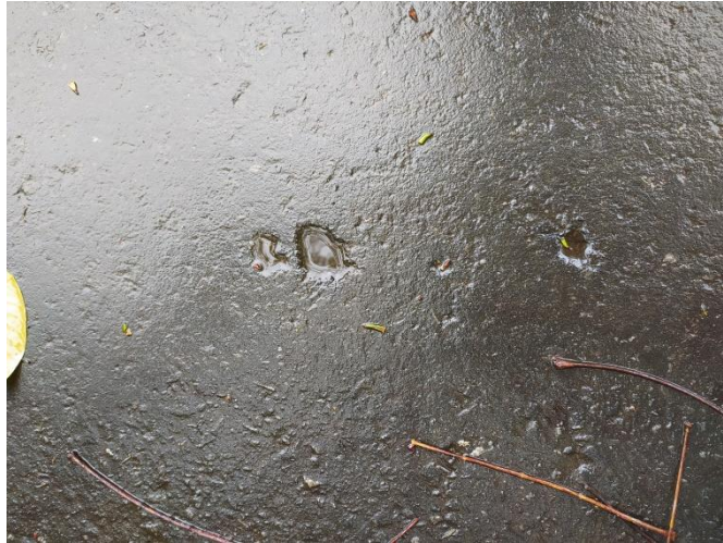
Figure 4.33: Section A - Raveling – dense mix asphalt (Low-Severity level)
