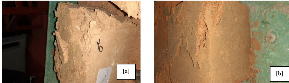
Figure 4-7 Corner cracks, horizontal[a], vertical cracks and diagonal cracks[b].
