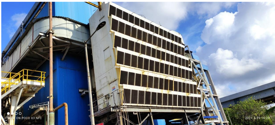
Figure 3.3 Gas Turbine Filter House (Original in Colour)
