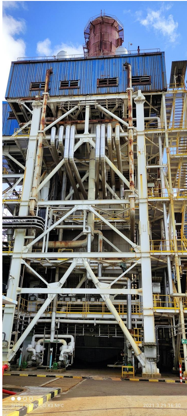
Figure 2.3 Heat Recovery Steam Generator (Original in Colour)
