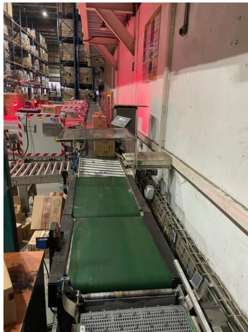
Figure 19: Newly designed and Built checkweigher Machine Unilever Horana Factory
