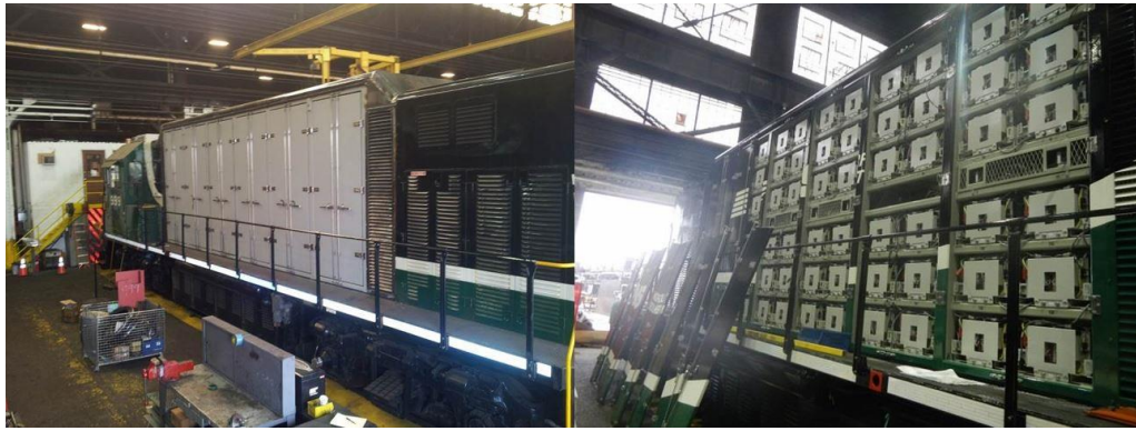
Figure 2.6: Installed battery ISO container and intra pack battery trays mounted on the NS 999 locomotive [29]
