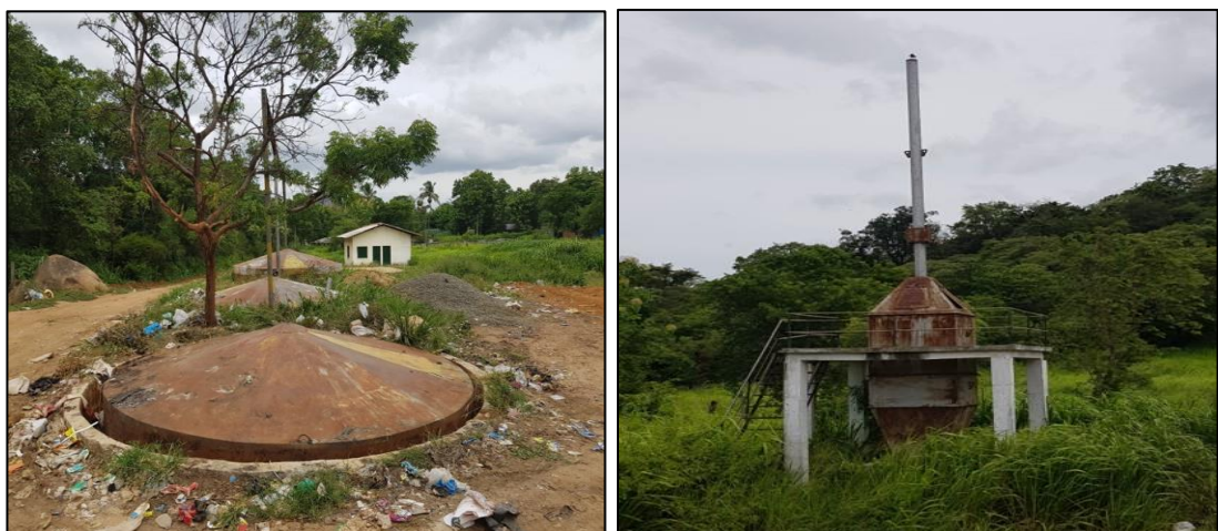
Figure 4.8: Underground tanks and other structures used for biogas generation
