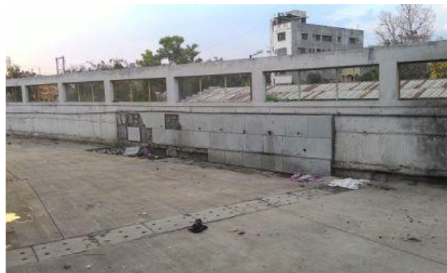
Figure 12: Deterioration of Paving and Compound Wall Photo courtesy: Ruikar Sharmishtha
