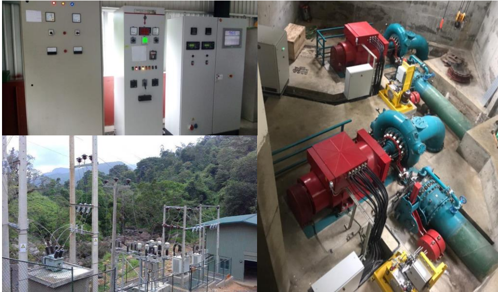
Figure 5: Electrotechnical equipment of Moragahaoya mini hydro power plant
