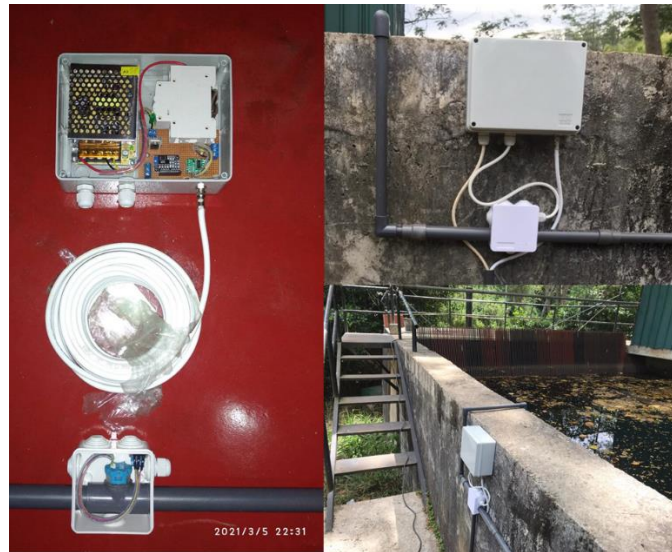
Figure 34 : installed hardware at the forebay.
