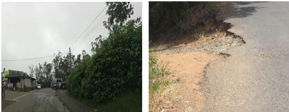
Figure 5.7. Excessive pavement edge drop-offs
