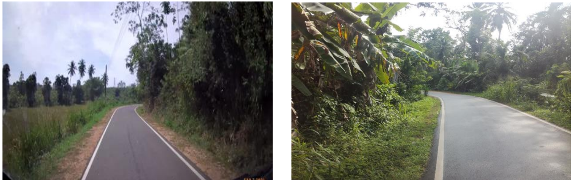
Figure 5.4. Road alignment, sight distance issues and lack of warning signs at curves
