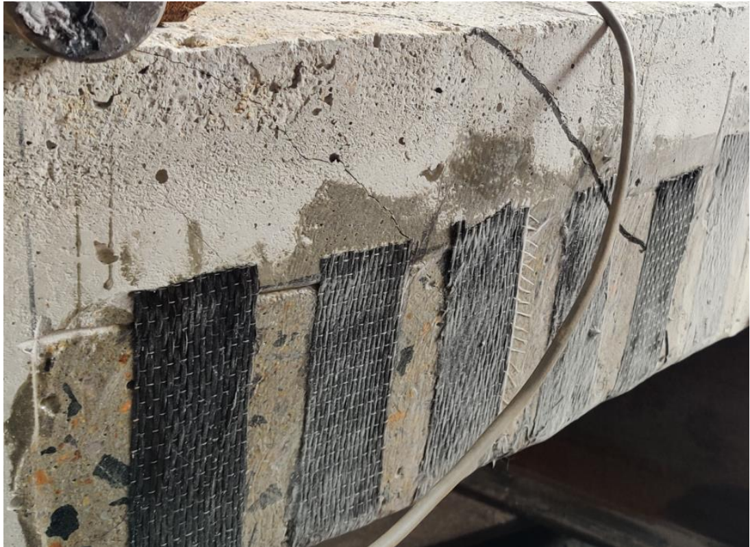
Figure 49: Shear cracks near CFRP wrappings
