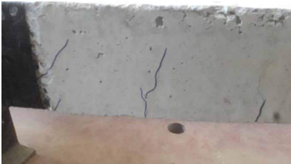
Figure 39: Shear cracks near CFRP wrappings
