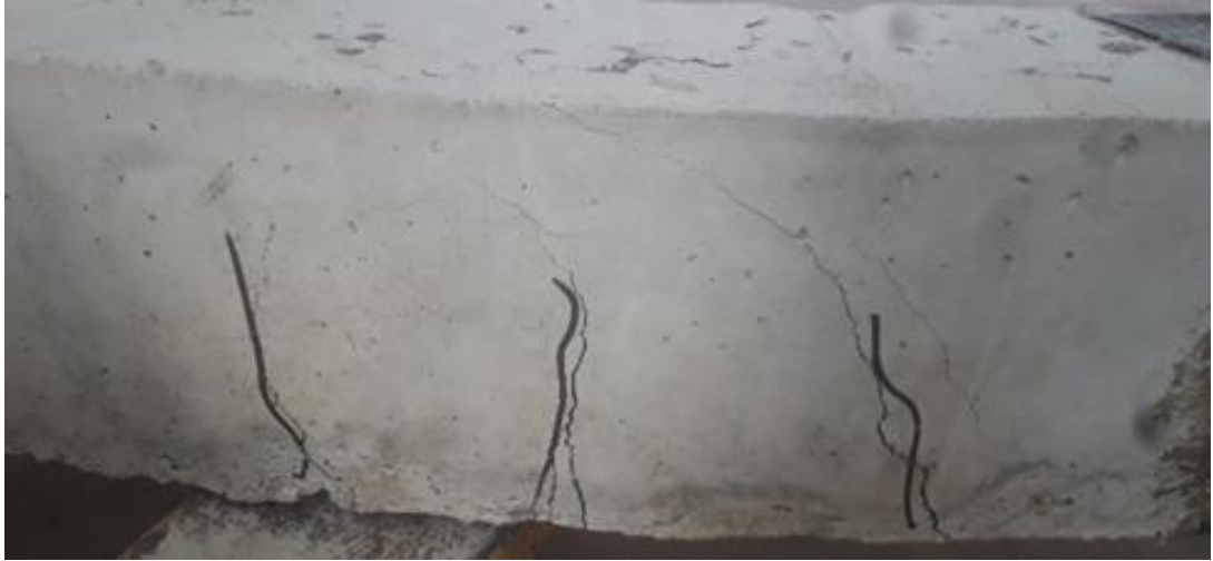
Figure 42: Cracks propagating with an inclination
