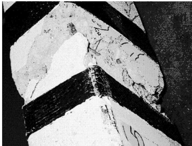
Figure 28: Spawling of concrete due to torsional failure (Ghobarah et al., 2002)
