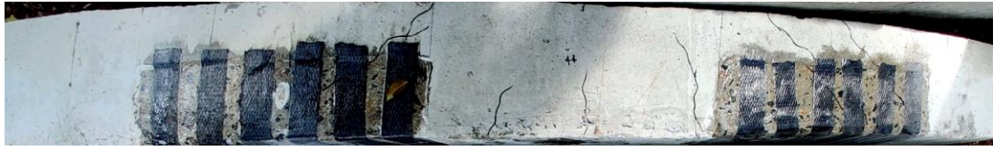
Figure 51: Flexural cracks at mid-span
