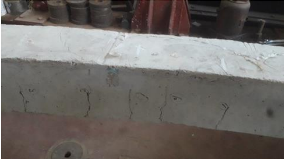
Figure 38: Initial flexural cracks
