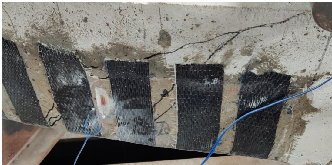
Figure 50: Cracks propagating with an inclination at loads beyond ultimate strength
