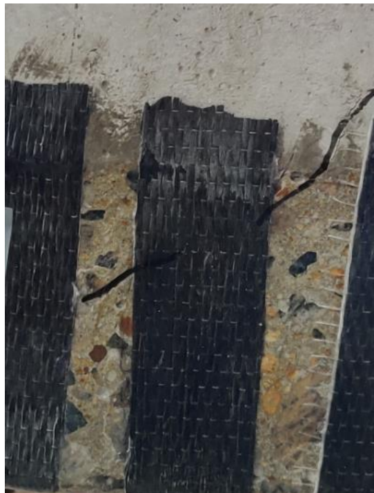
Figure 53: Shear crack induced intermediate debonding
