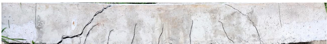
Figure 46: Cracks in a failed control beam
