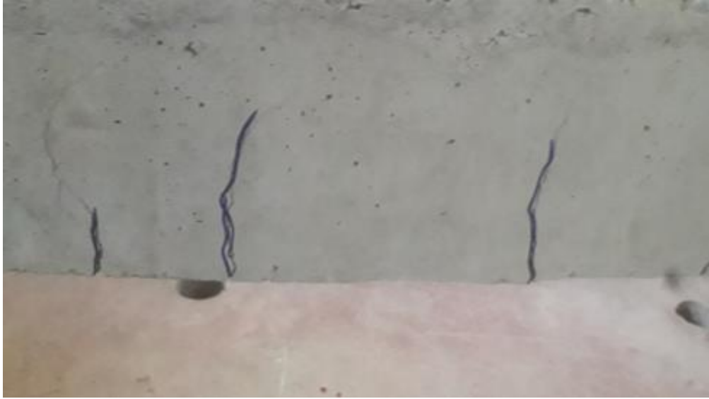
Figure 40: Cracks propagating with an inclination at loads beyond ultimate strength
