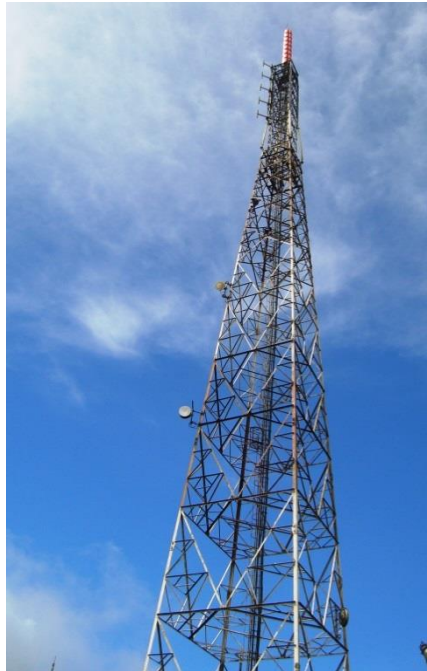
Fig. 2.4 – A typical self-supporting tower (at Kilinochchi SLT premises)
