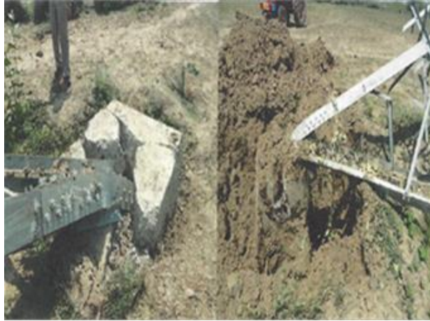
Fig. 2.16 – A collapsed directly embedded power transmission tower of 765KV Anta- Phagis S/C line in India (Standing Committee report on Failures of tower, CEA, India, 2016)
