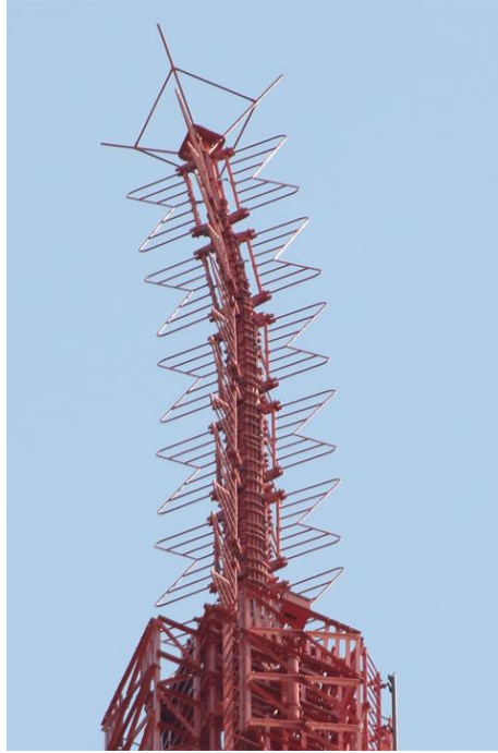
(b) Deformed top part of Tokyo tower after earthquake in 2011
