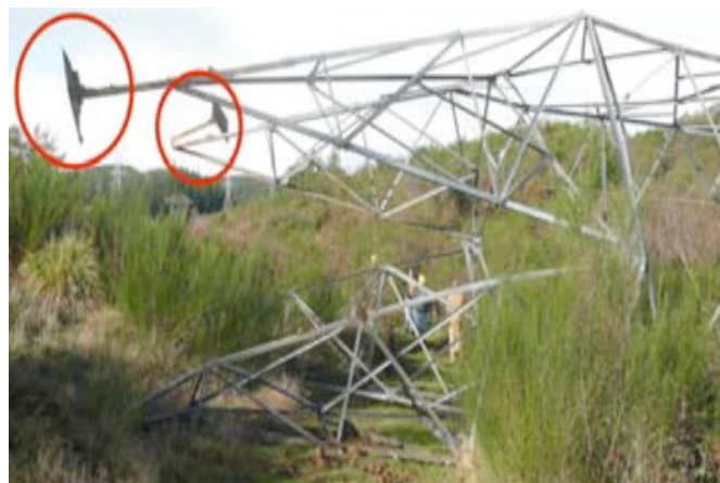
Fig. 2.15 –A failed power transmission tower at Washington, USA (Eidinger & Kemper, 2012)
