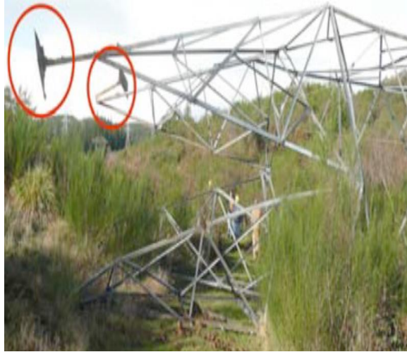
Fig 1.4 - Failed power transmission tower at Washington, USA in 1999 (Eidinger & Kemper, 2012)
