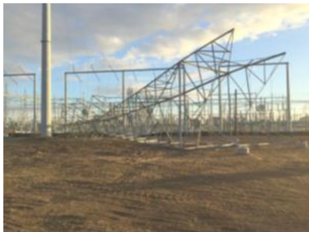
Fig. 2.17- Failed PG&E electric transmission tower located in Moss Landing, CA, 2015 (Brian and Rayan, 2015)
