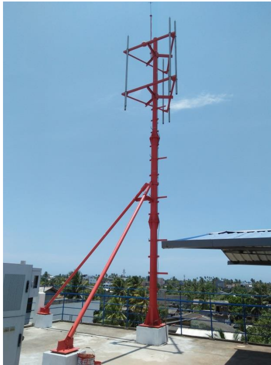
Fig. 2.3 – A typical pole with supporting struts (SLT rooftop tower at Galle)
