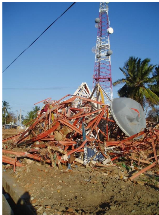
Fig 2.5 – Collapsed self supporting tower at Hambantota, Sri Lanka in 2004 Tsunami ( www.hikenow.net )
