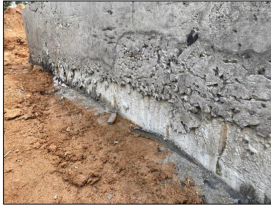
Fig. 4.8: Defects due to misalignment of formwork/mold
