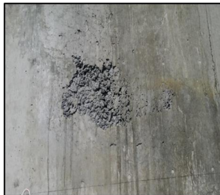
Fig. 4.9: Defects due to inadequate application of form oil
