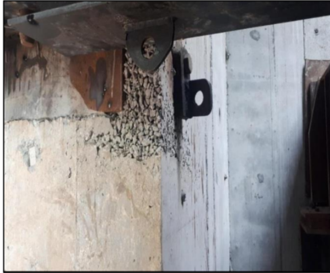
Fig. 4.6: Defects due to embedded parts-1
