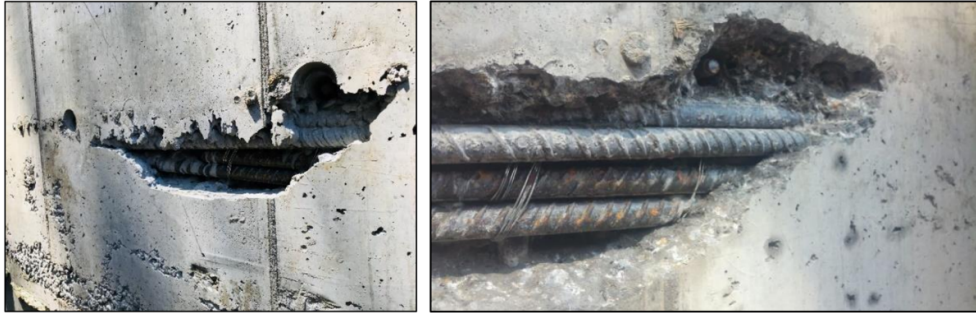
Fig. 4.2: Defects in a concrete wall due to reinforcement bar congestion.
