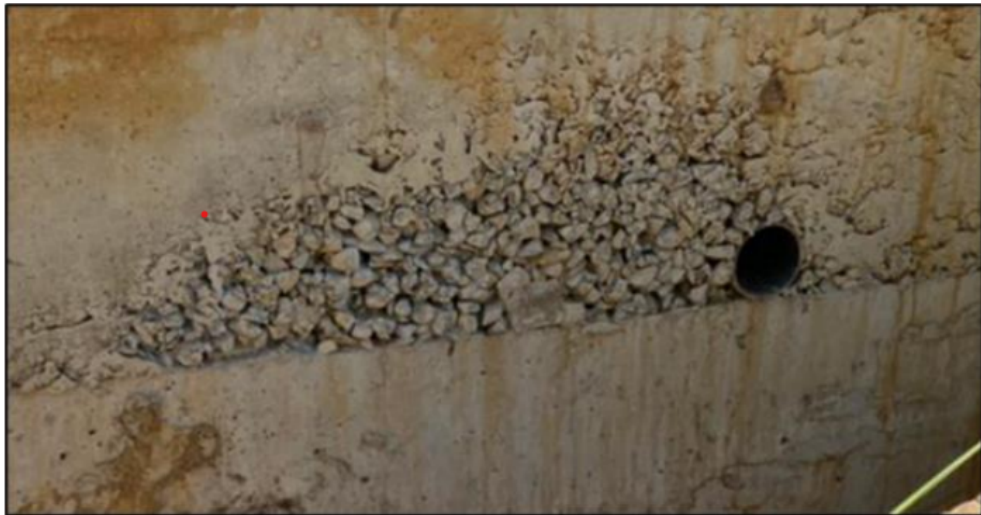
Fig. 4.1: Defects in a concrete retaining wall due to poor workmanship in compaction of concrete.
