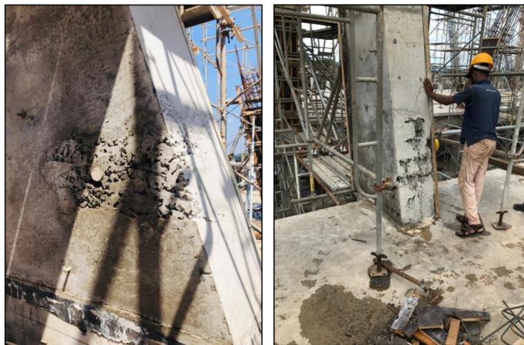
Fig. 4.3: Defects in an inclined concrete column.
