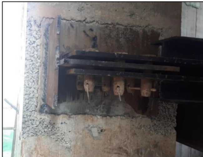
Fig. 4.7: Defects due to embedded parts-2
