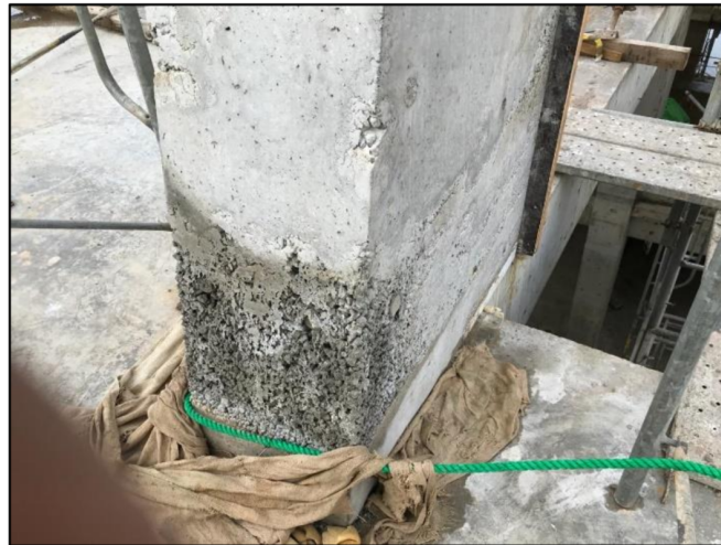
Fig. 4.5: Surface defects due to concrete slurry leakage.
