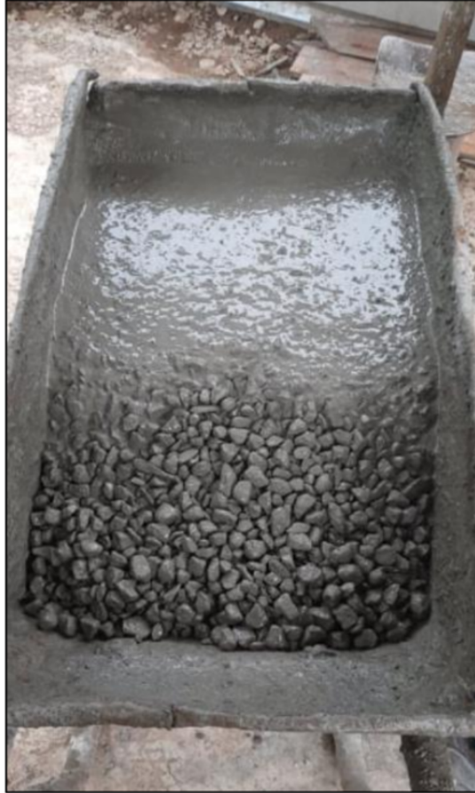
Fig. 4.10: Segregation of aggregates was observed from the ready-mix concrete.
