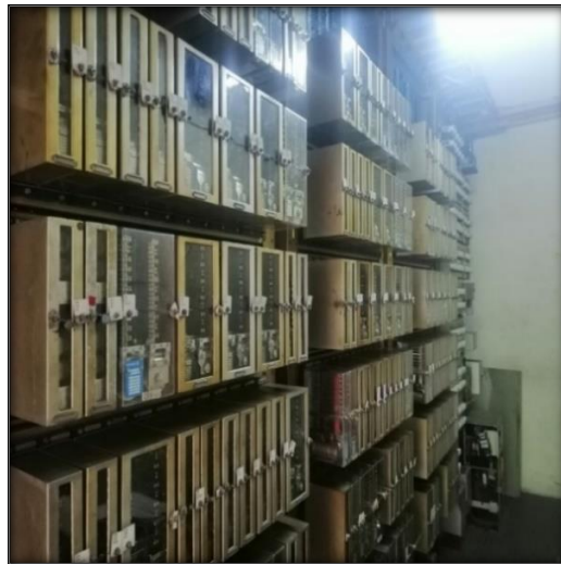
Figure 3 : Sri Lanka Railway Interlocking Relay House
