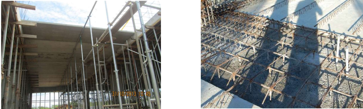
Figure 4.9: Supporting system and placing method on main beams of precast plank slab panels
